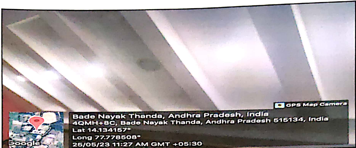
Fig: Power LED's bulbs in staff and office rooms
