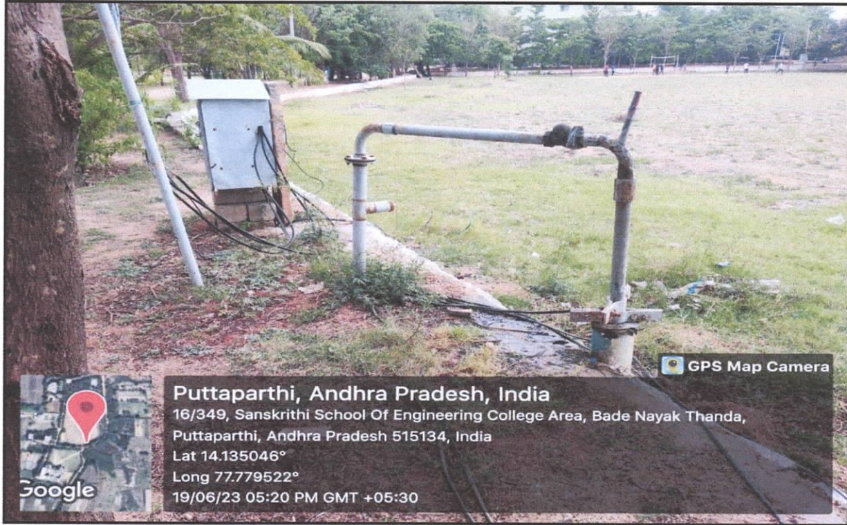
Fig: Bore well point near SSE Grounds
