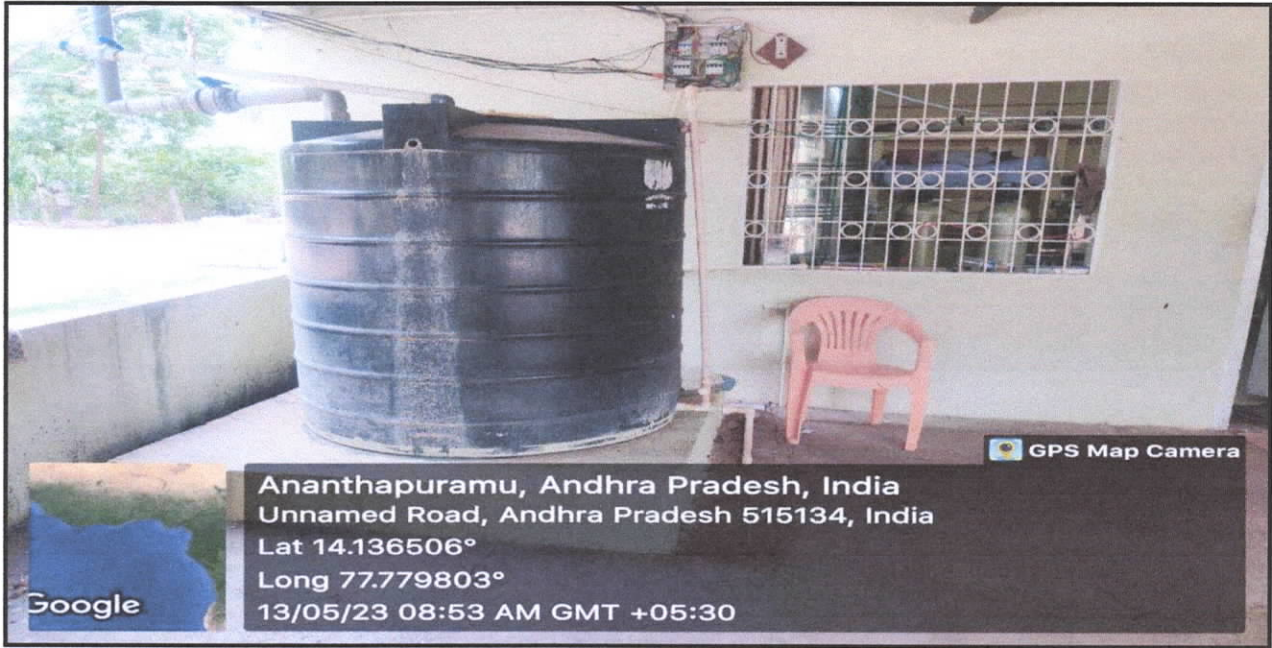
Fig: purified Water tanks for drinking
