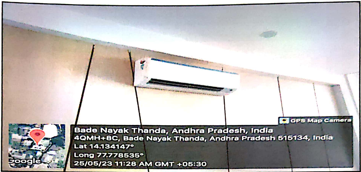
Fig: power efficient electronic devices in SSE staff rooms
